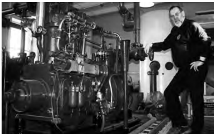
Ex-lighthouse Artificer Brian Johnson looking after one of the engines which power the foghorn.
